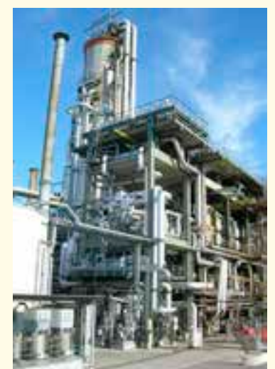
RD4 plant for OMV at Schwechat, Austria, 2010
